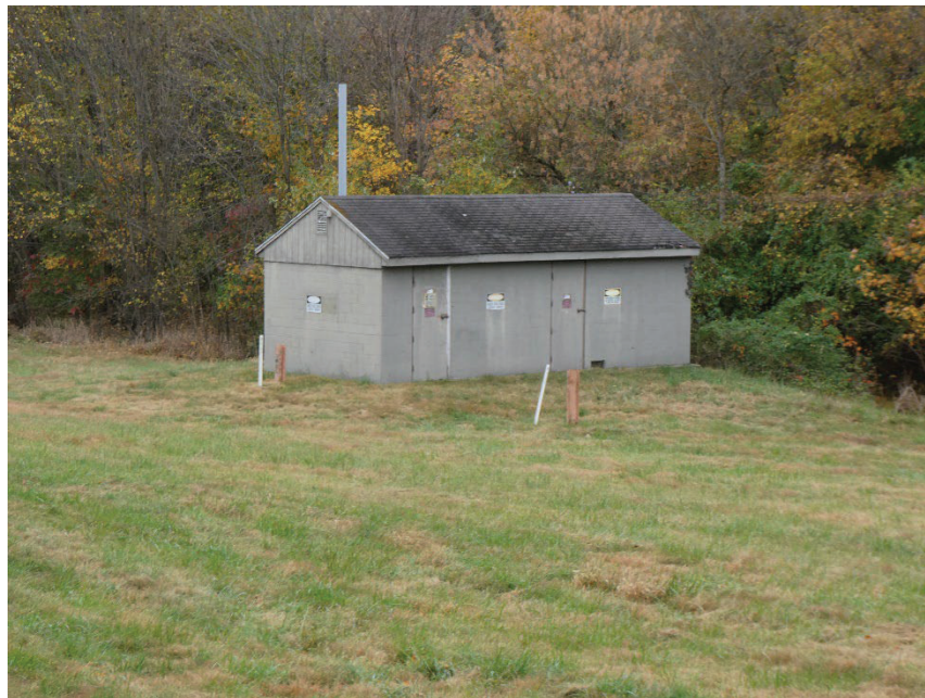
The electrical housing for the former landfill gas venting system. (Removed March 2023)
