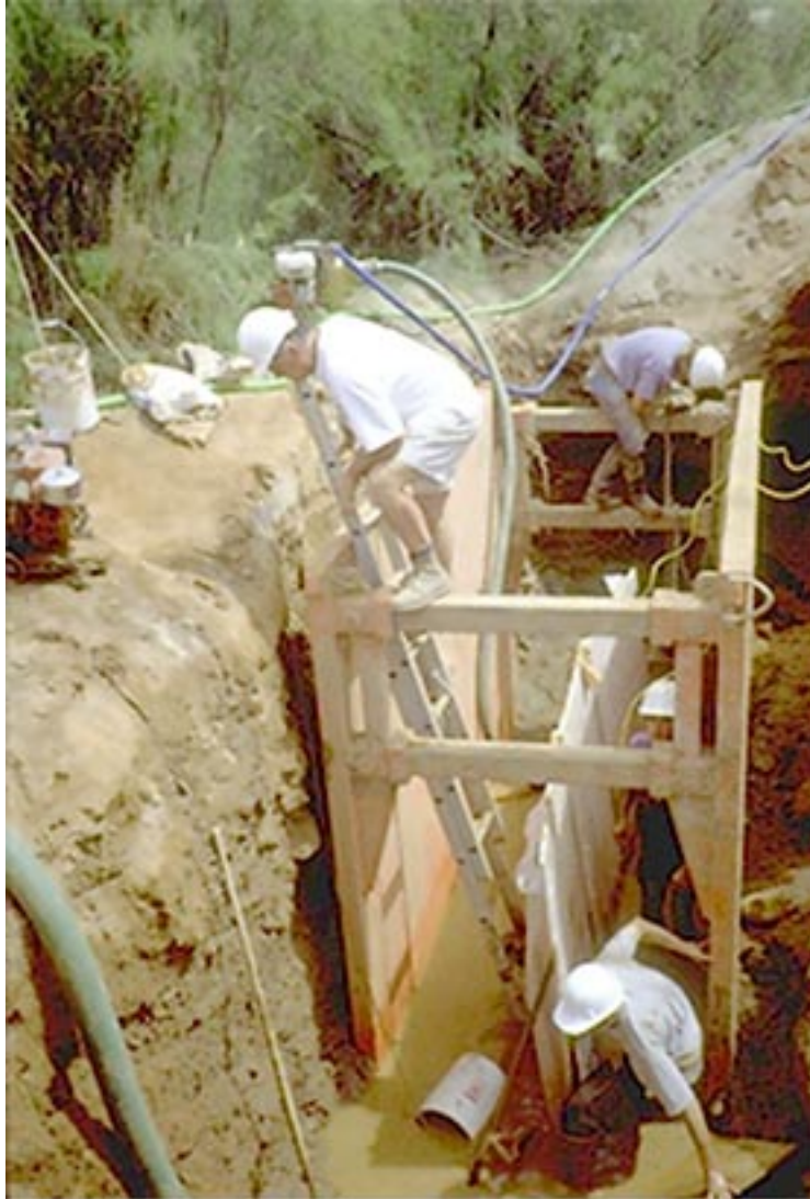
Figure 5.1. Trench box used to protect workers during installation of the PRBs at Fry Canyon, Utah.
