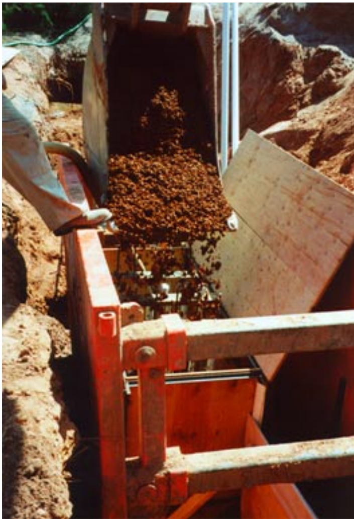
Figure 5.2. Placement of AFO barrier material into the gate structure of the permeable reactive barrier, Fry Canyon, Utah.
