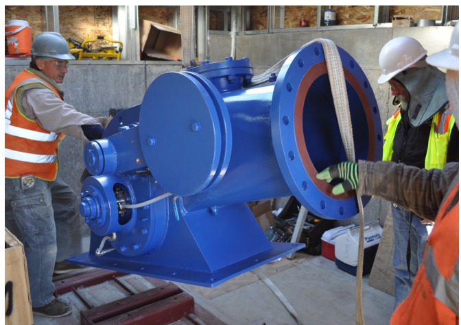
Installation of hydroelectric equipment at the Summitville Mine site in Colorado in 2010. Source: EPA
