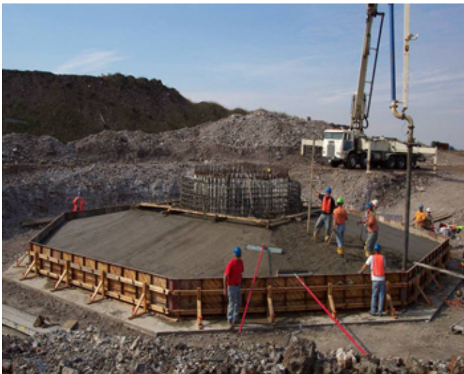
Construction of a wind turbine foundation for the Steel Winds project. Source: First Wind
