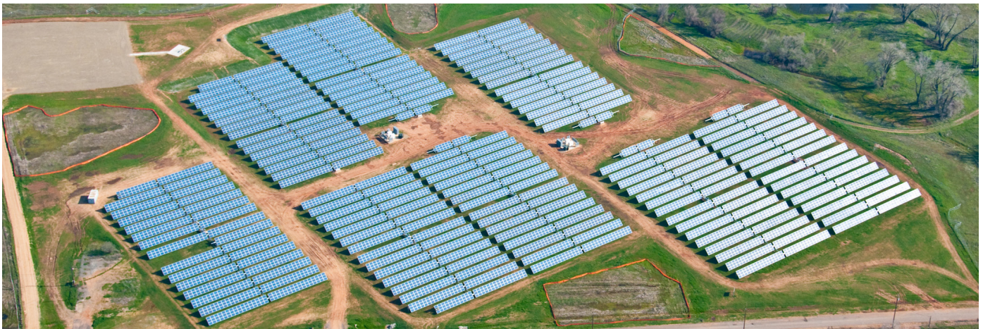
Aerojet's solar farm helps power the site's ground water cleanup and is one of the largest industrial installations in the United States. Source: Aerojet
