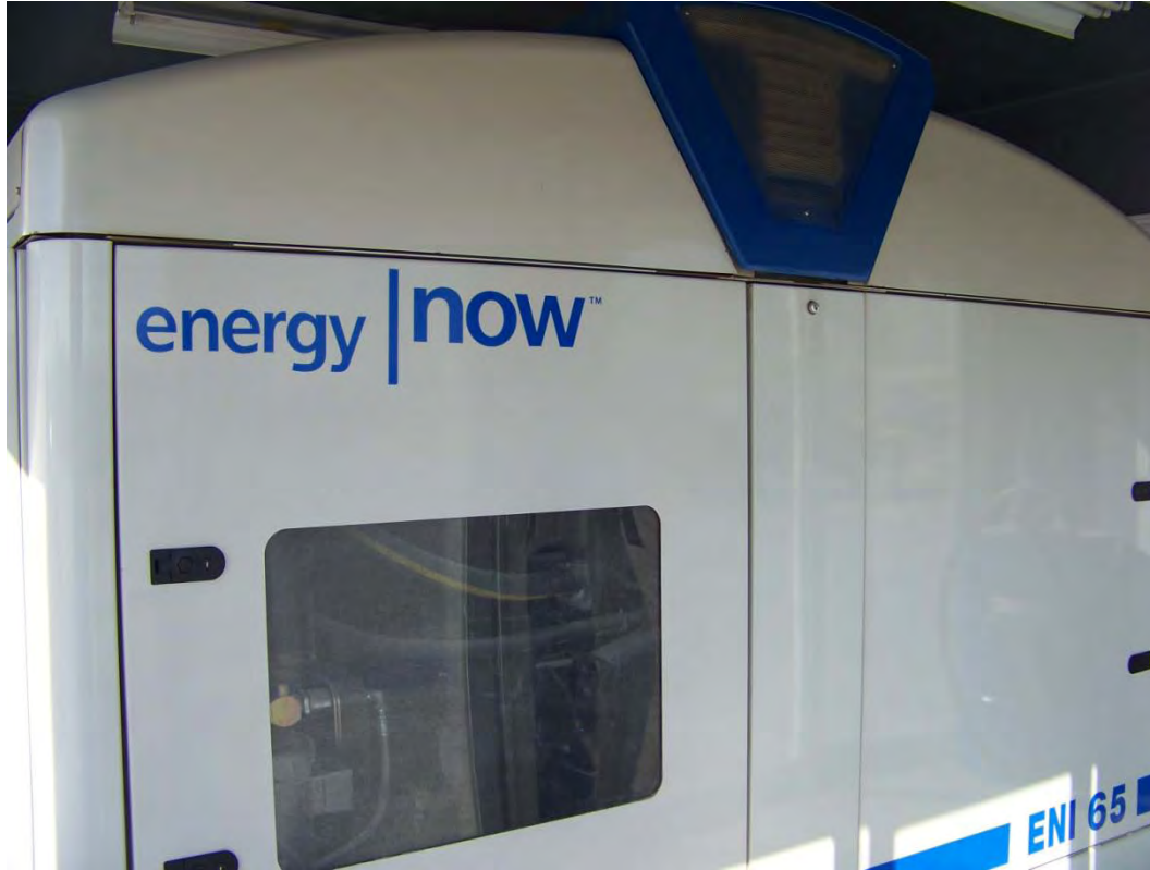
65 kW IPower Energy Systems Generator
