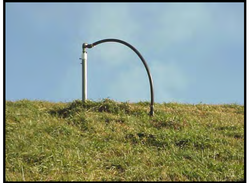
Gas Well at South Side
