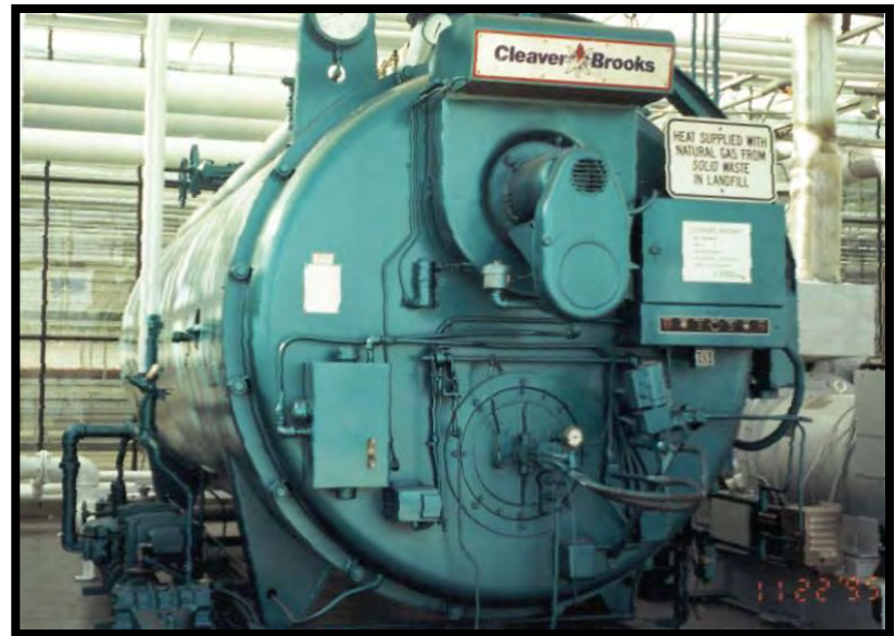
Cleaver Brooks Boiler at Greenhouse
