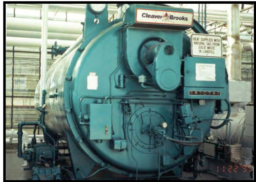
Cleaver Brooks Boiler at Greenhouse
