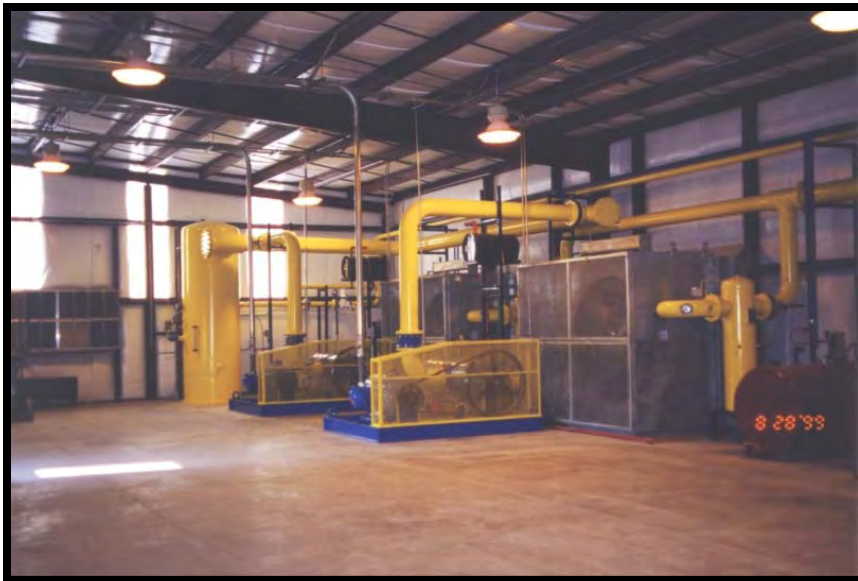
LFG Compression and Treatment Facility
