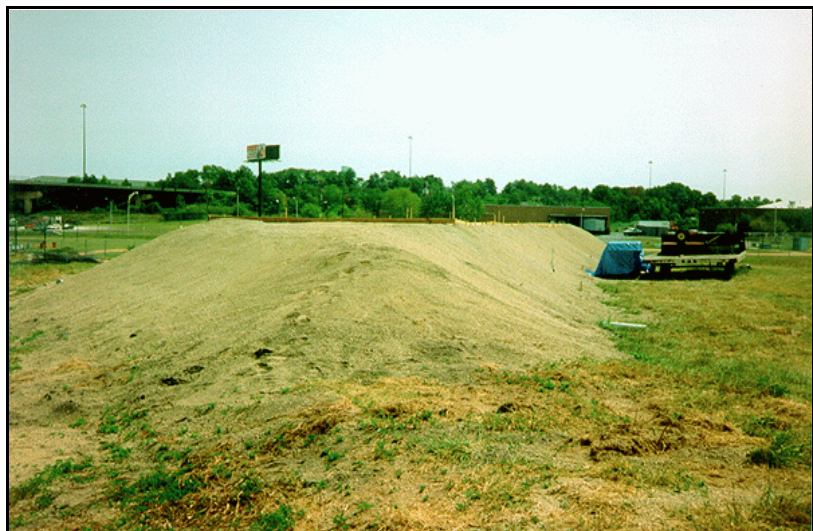
Construction of the foundation for the golf tees for the driving range built on top of the Kane & Lombard Street Superfund site in Baltimore, Maryland.
