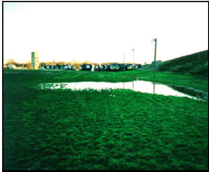
A soccer field built on a portion of the Fairfax County Municipal Landfill in Virginia illustrates the need to address settlement, which can cause depressions in the cap that can lead to drainage problems and poor field conditions.
