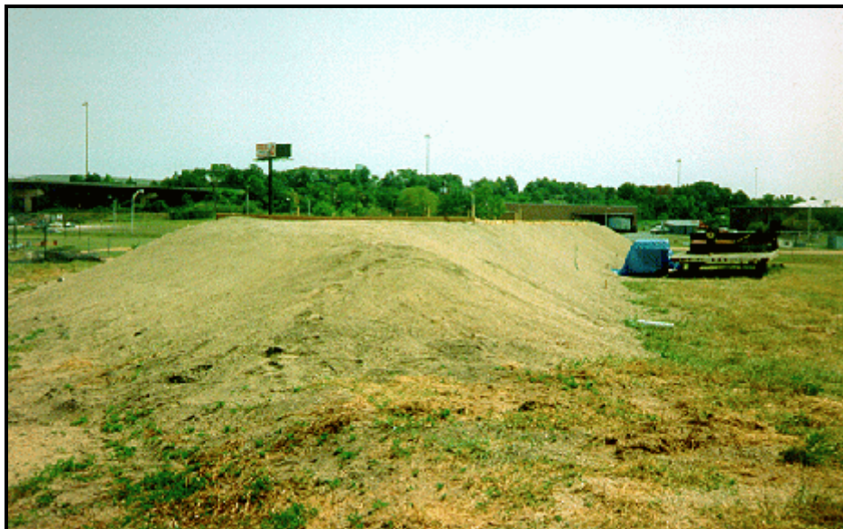
The foundation for the golf tees is constructed for the driving range that was built on top of the Kane & Lombard Street Superfund site in Baltimore, Maryland.
