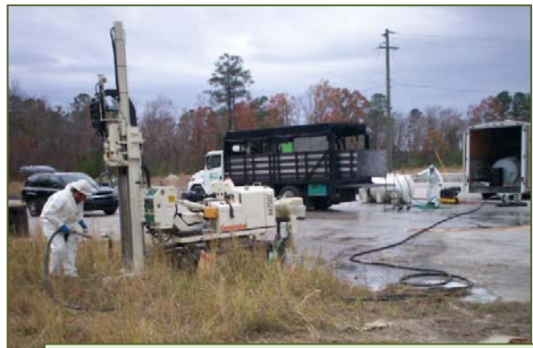
Integrated planning of bioremediation activities at Marine Corps Base Camp Lejeune enabled injections of emulsified vegetable oil and sodium lactate in four borings to be completed within only one week, which reduced field redeployment and associated fuel use.
