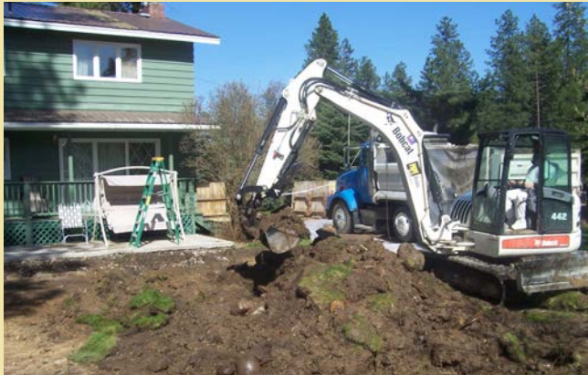
EPA and MDEQ remove asbestos from about 150 properties each year.
