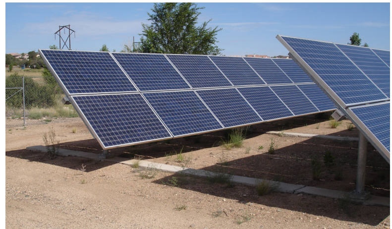
Example of a PV array at the nearby Embry-Riddle Aeronautical University APS Solar Power Plant
