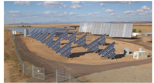
Arizona Public Service’s (APS’s) 3.5 MW Prescott Airport Solar Plant includes tracking PV and concentrating PV arrays. Source: APS
