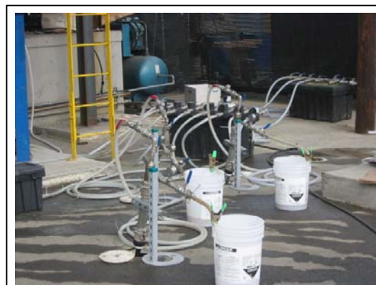
Figure 1. ISCO Application Wells
