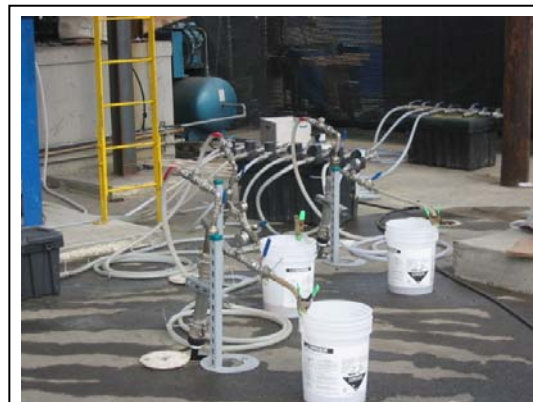
Figure 1. ISCO Application Wells
