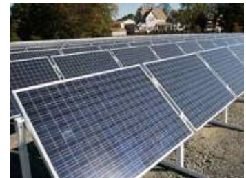
Top: Tracking PV panels follow the sun to allow for increased solar capture. Bottom: Fixed axis PV panels aligned to be south facing.
