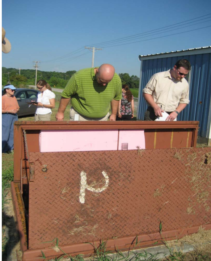
The bulkhead providing access to the soil washing system with pumping station in the background
