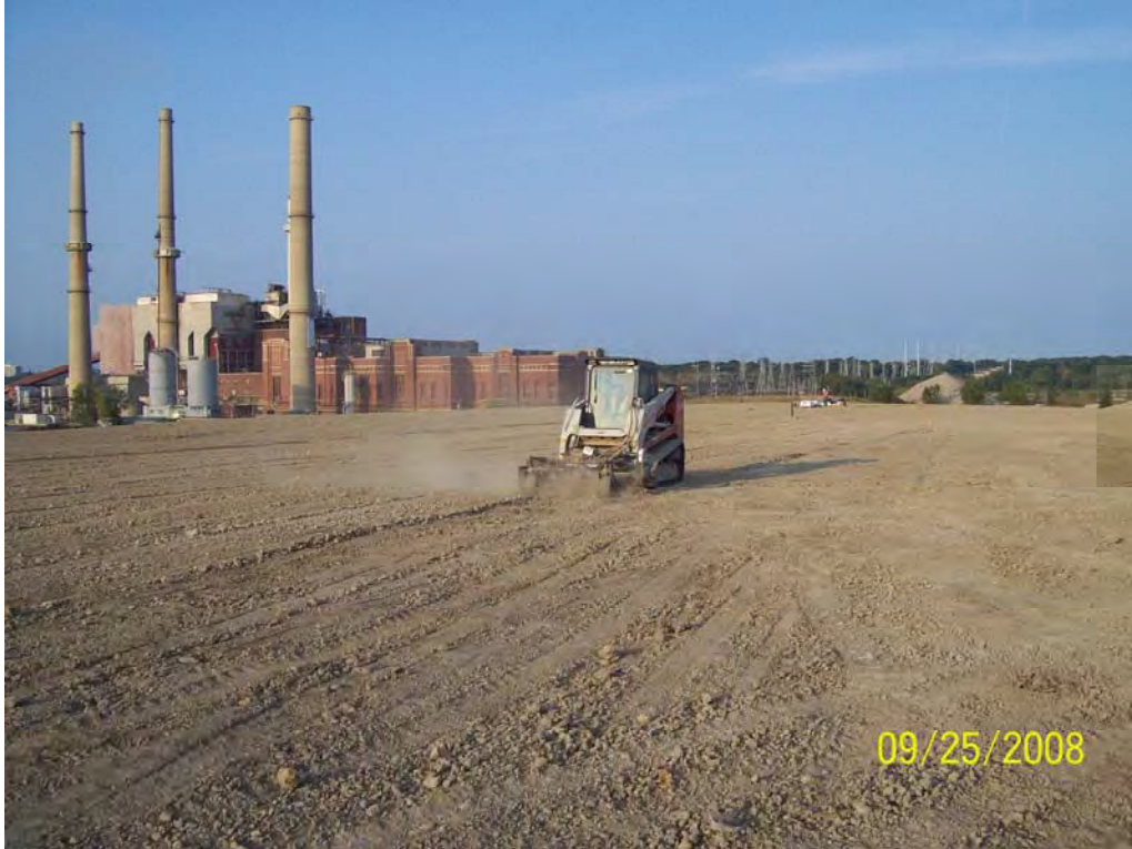
Photograph No. 22 _____ September 25, 2008 Photographer: Chris R. Goffard Signature: Chris R. Goffard Scarifying the surface prior to seeding on Area 1 Final Cover. Viewing west.
