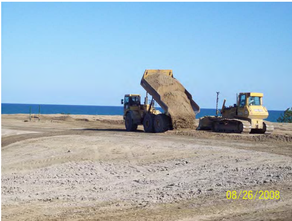
Photograph No. 6 Photographer: Chris R. Goffard Sand drainage layer material placement on Area 1 Final Cover. Viewing east. Signature: Chris R. Goffard August 26, 2008
