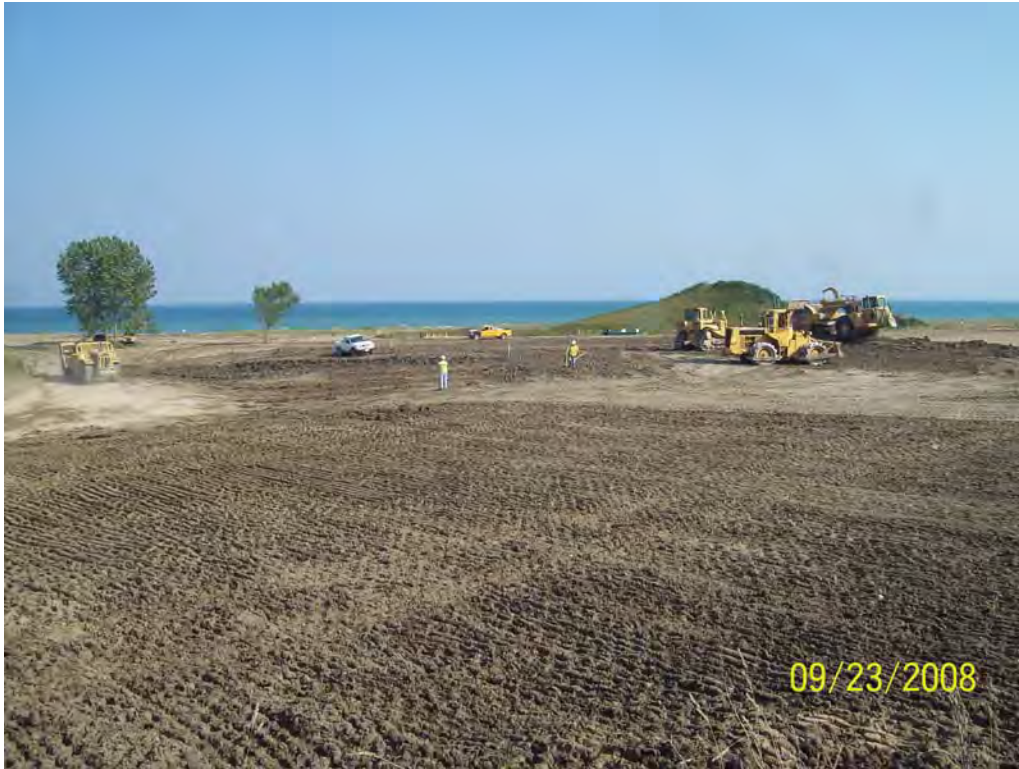
Photograph No. 19 Photographer: Chris R. Goffard Placement of protective layer material on Area 2 Final Cover utilizing Caterpillar 627 scrapers. Viewing east.
