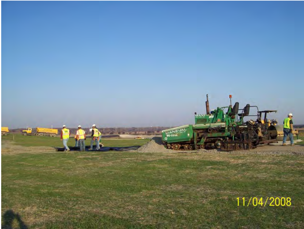
Photograph No. 27 _____ November 4, 2008 Photographer: Chris R. Goffard Signature: Chris R. Goffard Placement of woven geotextile on the access road for Area 1 Final Cover. Viewing west.
