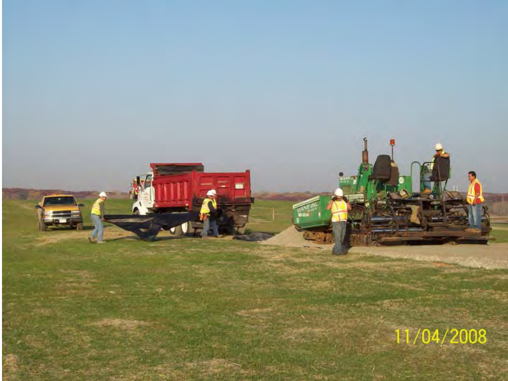
Photograph No. 28 _____ November 4, 2008 Photographer: Chris R. Goffard Signature: Chris R. Goffard Placement of CA6 aggregate material on the access road for Area 1 Final Cover. Viewing west.
