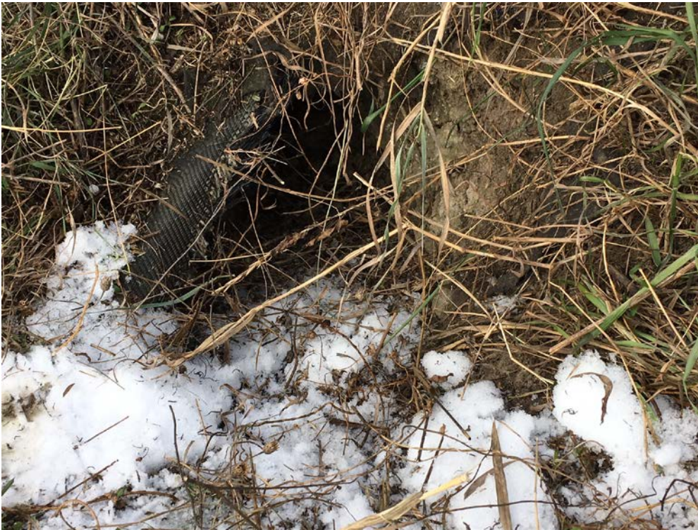
Photo showing animal burrow in northern berm of Settling Basin. Burrow to be repaired and material repaired.
