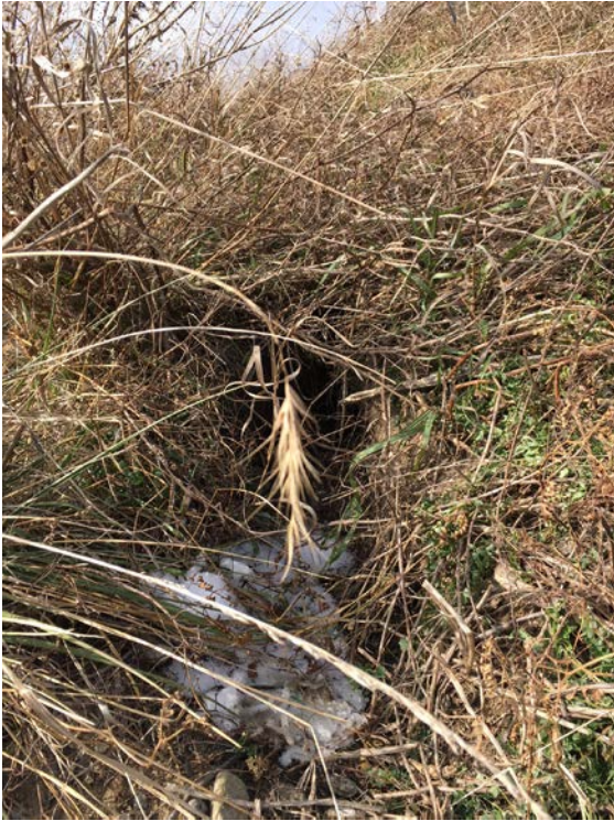
Animal burrow within Settling Basin berm.
