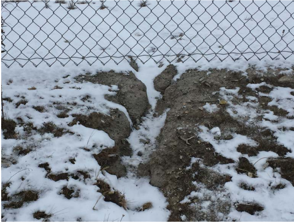
Figure looking north at OU8 / Site 6. Minor erosion (6-inch) underneath fence to be repaired in Spring.
