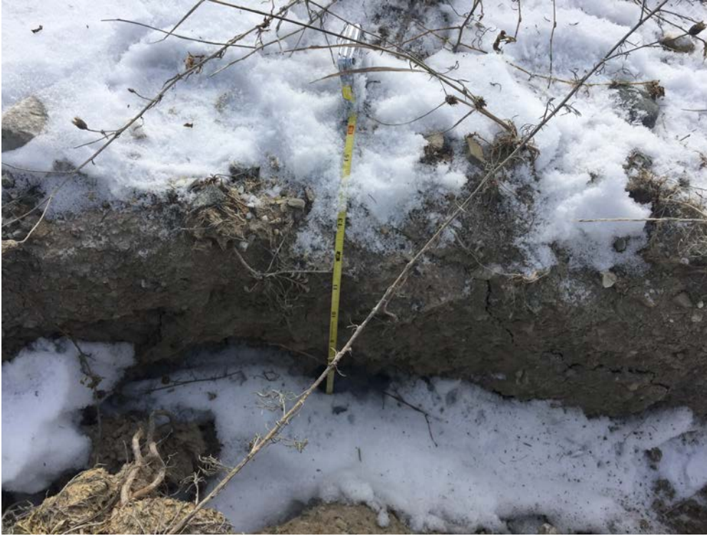
Stormwater erosion gully in western berm of Settling Basin. Gully is approximately 13-inches deep. Gullies are typical along berm face, and are scheduled for repair.
