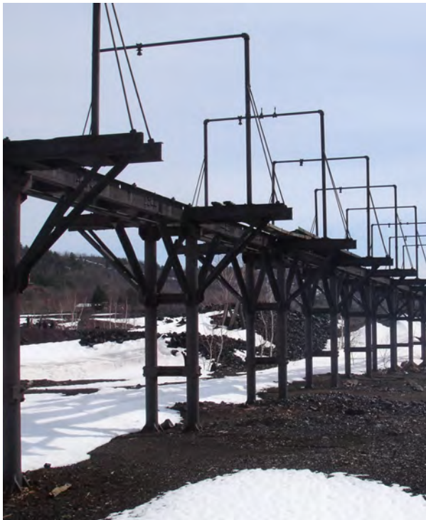
Overhead rail trestles are one of the historic features at Quincy Smelter. Source: EPA.
