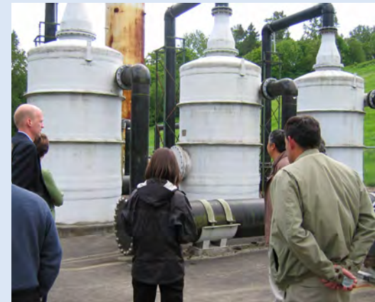
Groundwater treatment system
