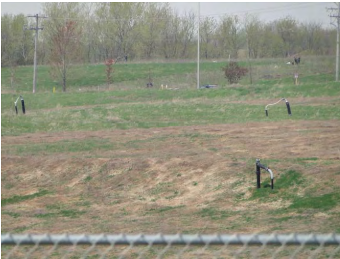
Gas extraction wells are scattered across the 1978 and 1985 Landfills
