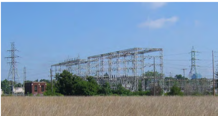
Consumers Energy owns the transmission lines that traverse the site (top), as well as the Wealthy Street electric substation located adjacent to the site (bottom).
