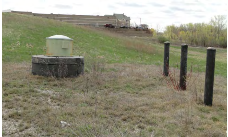
Leachate collection system and monitoring wells in the foreground, Sam's Club commercial retailer in the background.
