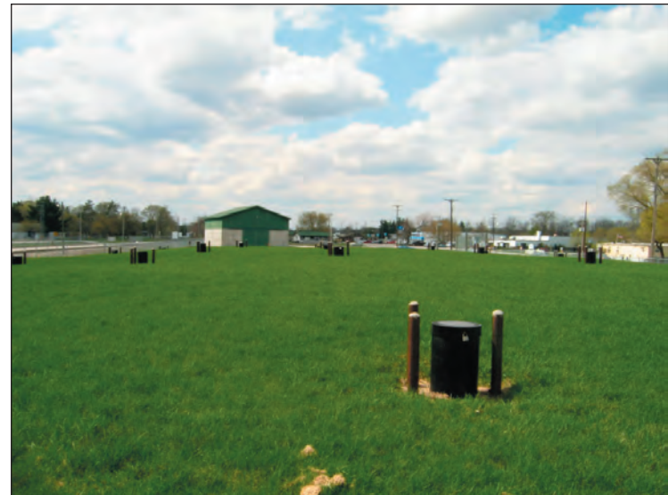
Containment Cell at the Ex-Cell-O Property
