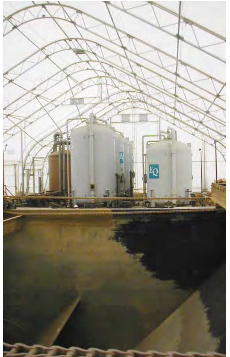
Interior of Water Treatment Facility at the Velsicol Corp. Superfund Site (2003)
