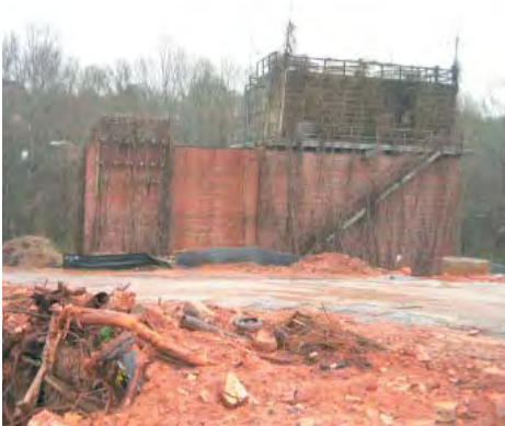
View of Power Station #6
