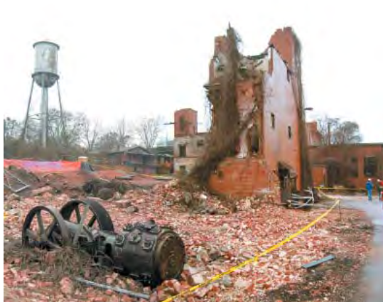
View of Water Tank, Brick Debris, Mill Equipment, and Remnant Mill Building #3
