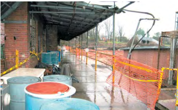
View of Covered Walkway / Concrete Porch Adjacent to Buildings A, B, and C
