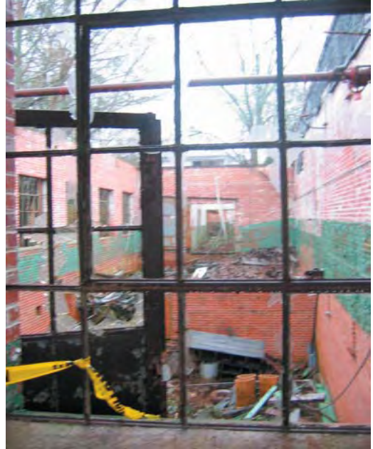
View from Covered Walkway, Looking into the Area Between Buildings B and C
