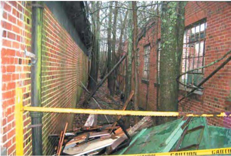
View of Vegetation Growing in between Buildings B and C
