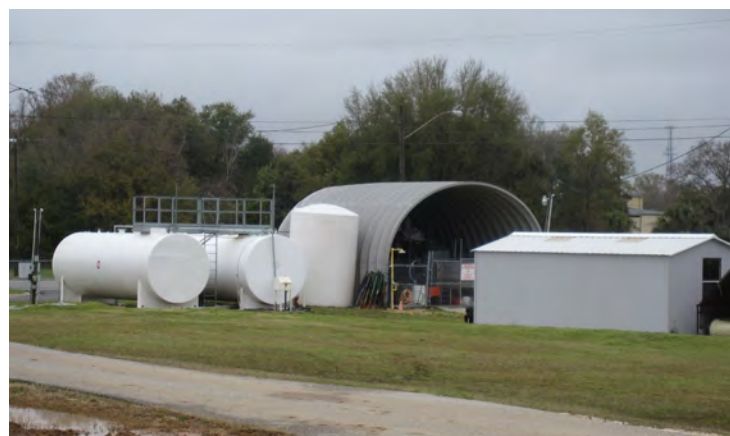
Ground water treatment compound at the ACW Site.
