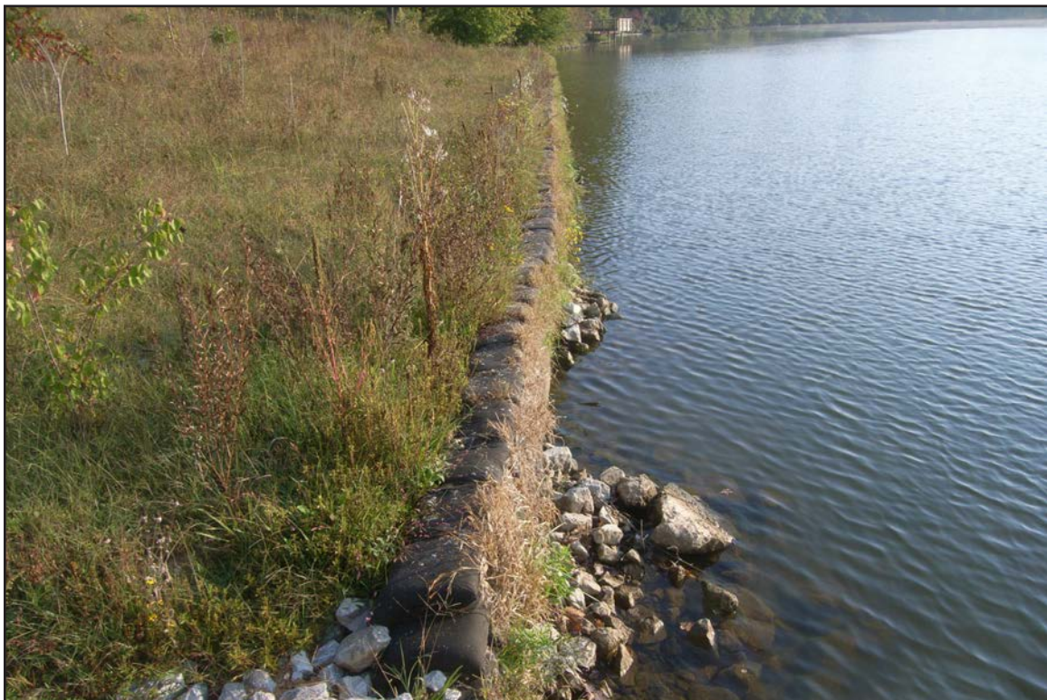
12B – Vegetative slope stabilization - Established wall vegetation. October 2, 2014.
