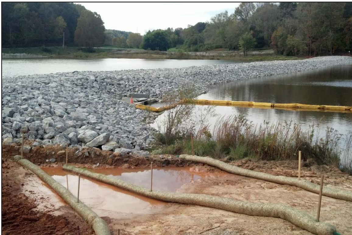
13B – Weir 2 at the North Berm dike in the North Embayment. October 20, 2014.
