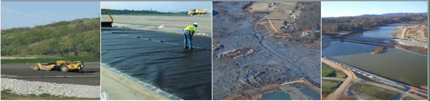
Left to right: Cleanup work at the site, cap installation, and a before and after of the Middle Embayment area.
