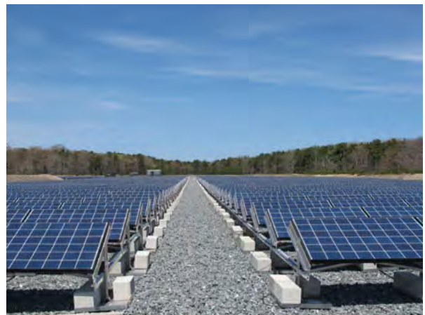
Figure 6: A ballast-weighted system using pre-cast concrete slabs in Barnstable, Massachusetts (source: NEXAMP)
