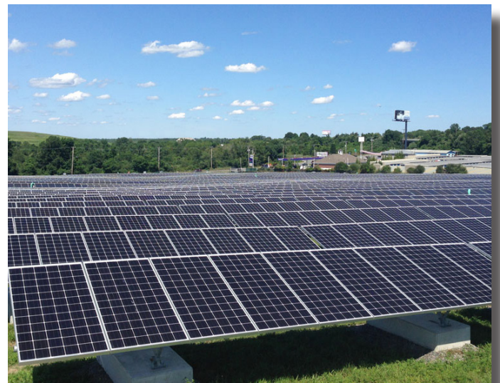
The 1.8-megawatt Sullivan's Ledge solar facility.
