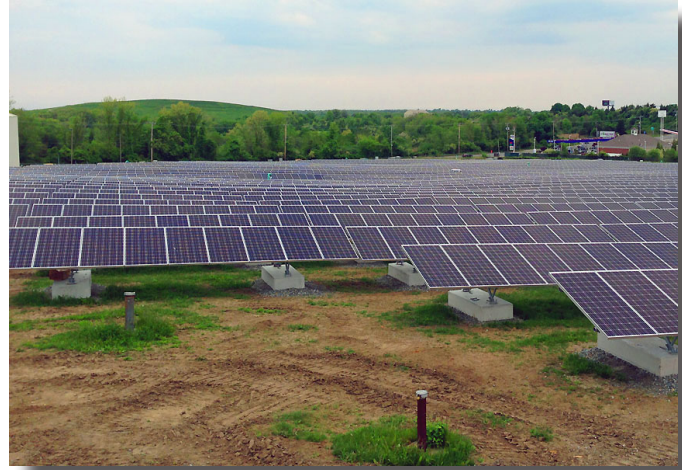
Installed solar panels at Sullivan’s Ledge.
