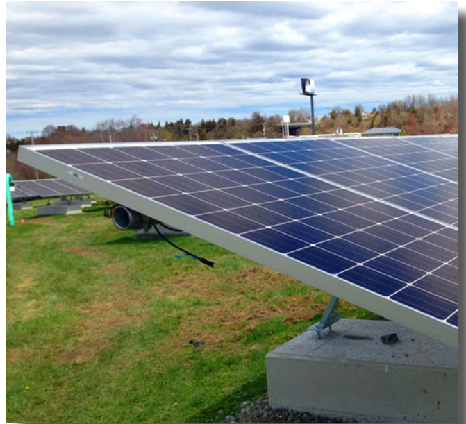
Installed solar panels at Sullivan’s Ledge.
